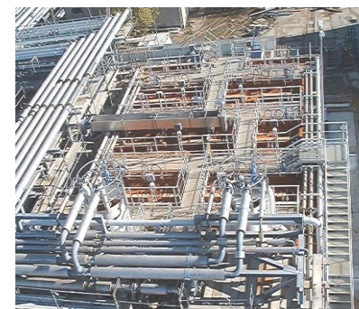
HDS plant (multi-stage neutralization)
